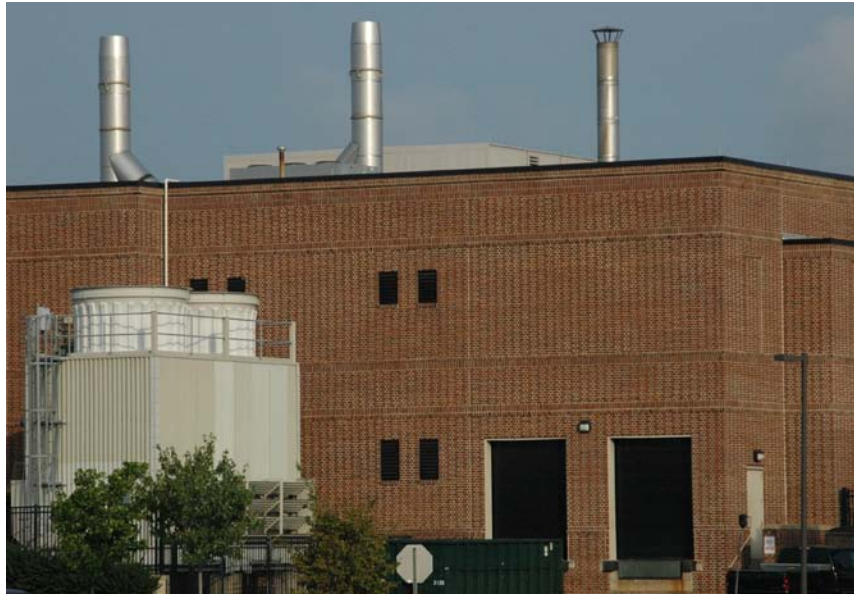
UVC-treated water produced by the air handlers during cooling season at the Delaware Biotechnology Institute on the campus of the University of Delaware is clean enough to be pumped into the cooling tower.
