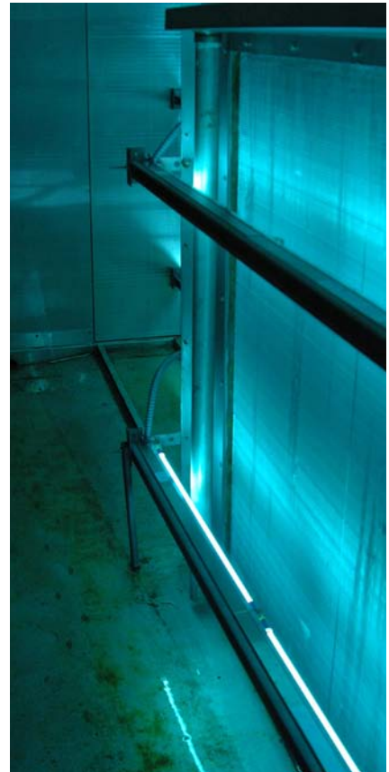
UVC lights shine on one of the air conditioning coils at the Delaware Biotechnology Institute.
