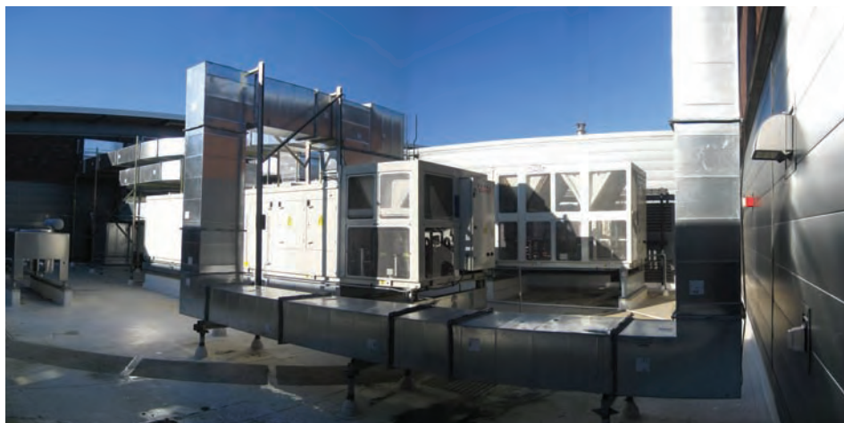
Heating and cooling for the Sammamish, Wash., city government building is provided by two packaged rooftop air-handling units designed by Petra Engineering. Both VAV units are equipped with DX and hot water coils, and can provide 100 percent economizer cooling.
